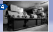
500 kVA Diesel CPS System
